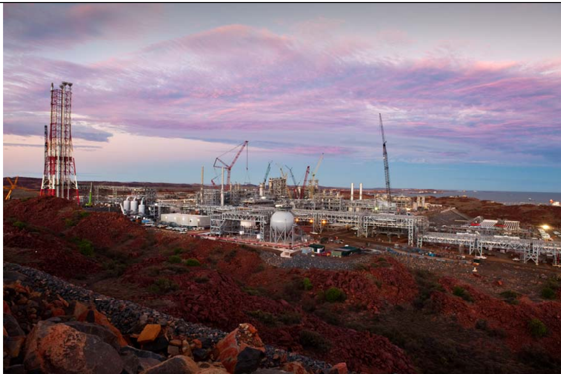
Plate 6: The Pluto LNG Project is transitioning from the construction phase to commissioning during 2010.
